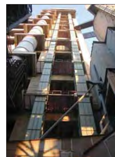
Giant Beumer belt bucket elevator recently installed at an Indian cement plant
