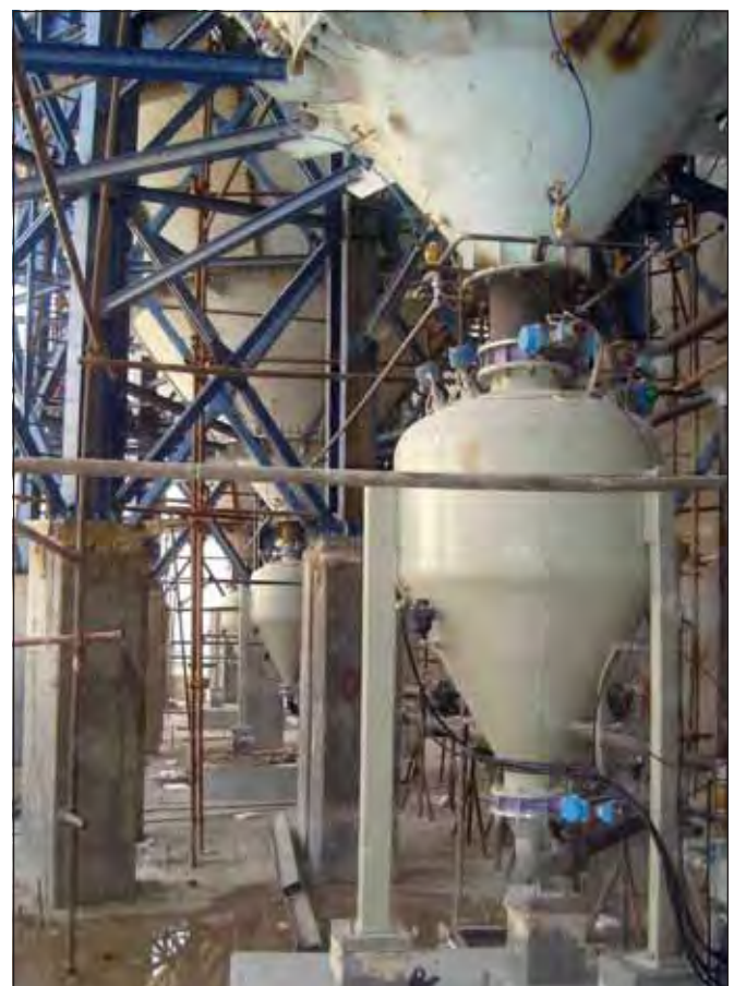
Air-Tec System pneumatic conveying transporters at the construction site of the Karun IV dam in Iran
